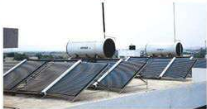
Solar Water System
