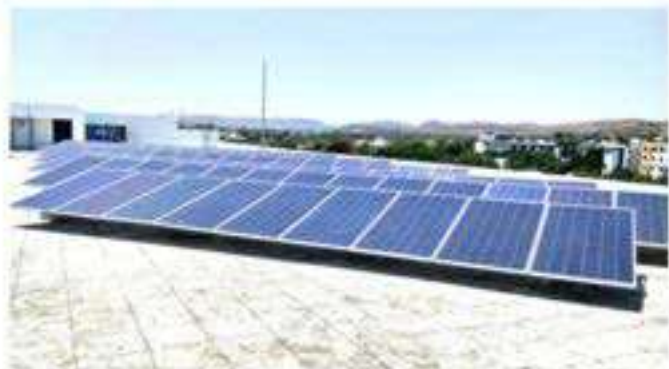
Solar roof top Photo - Voltaic Project
