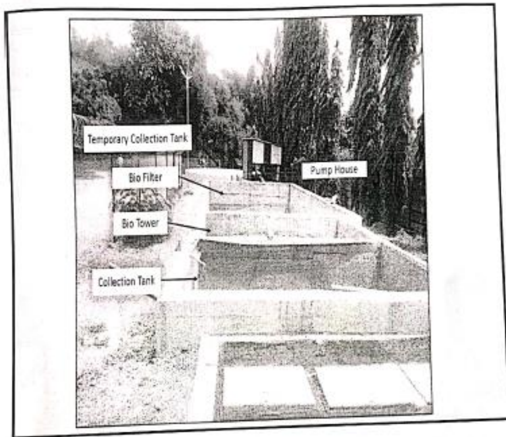
Figure: 3 Photograph showing Sewage Treatment Plant
