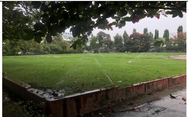
Sprinkler System for lawn
