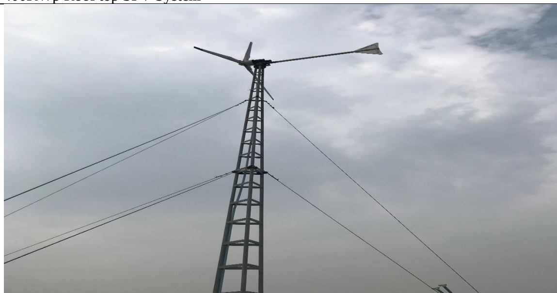
5KW Wind Generator
