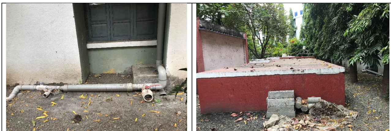
Rain Water Harvesting System
