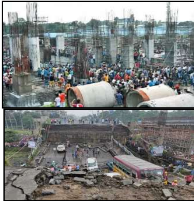
Fig.7: Kolkata- Joka Esplanade Metro project and collapsed bridge
